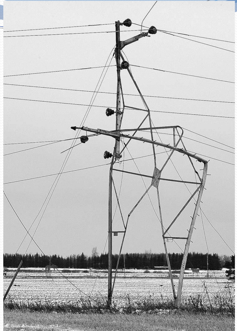
Damaged power lines in eastern Manitoba on October 6, 2012
